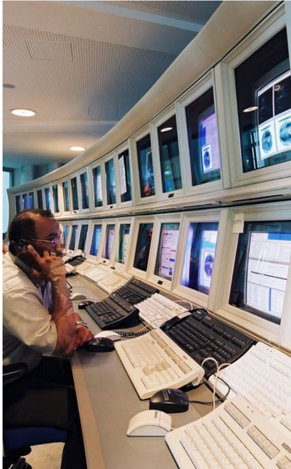
MTP Control Centre
